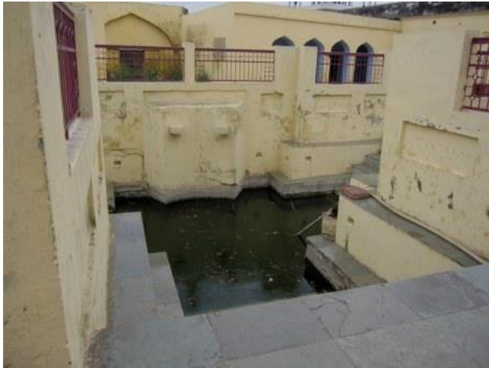
Figure 47. Nakka Kuan in a dilapidated condition
